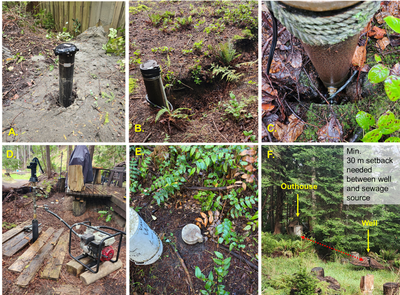
Figure 29. Savary Island well protection observations. A. New well with subsidence and unfilled annular space surrounding the casing after drilling (must be filled in with sealant and regraded). B. An unfilled trench where water lines were installed or C. annular space left open after installation of pitless adapter (water line) below ground. Both provide a preferentially pathway for contaminants to infiltrate toward the well and into the aquifer. Surface seal should be restored, trenches filled and area around well regraded to protect the well. D. Gas generator with no spill pan less than 3 m from well. An accidental spill could contaminate the well and aquifer. E. A low casing stickup (<0.3 m) increases risk of flooding, vermin or contaminant entry into a well. F. A well that is located close to a sewage source is at higher risk of contamination.
