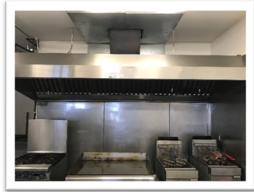
exhaust/fire suppression hood with roof fan
